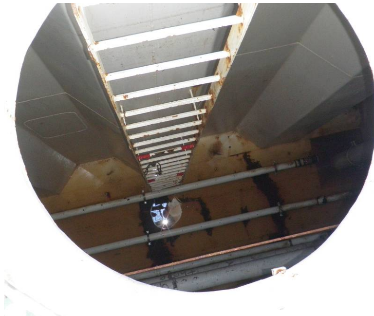
Figure 8. A holding tank, empty
